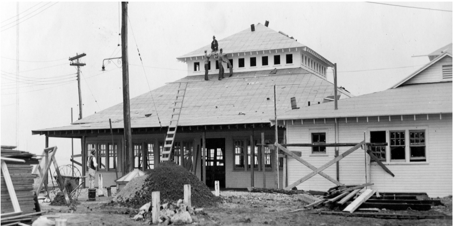
Construction of the Colony Inn. See ad below for the finished product offering dining, dancing, and entertainment.
